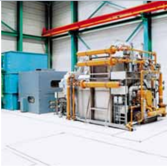
4 Steam turbine generator set
