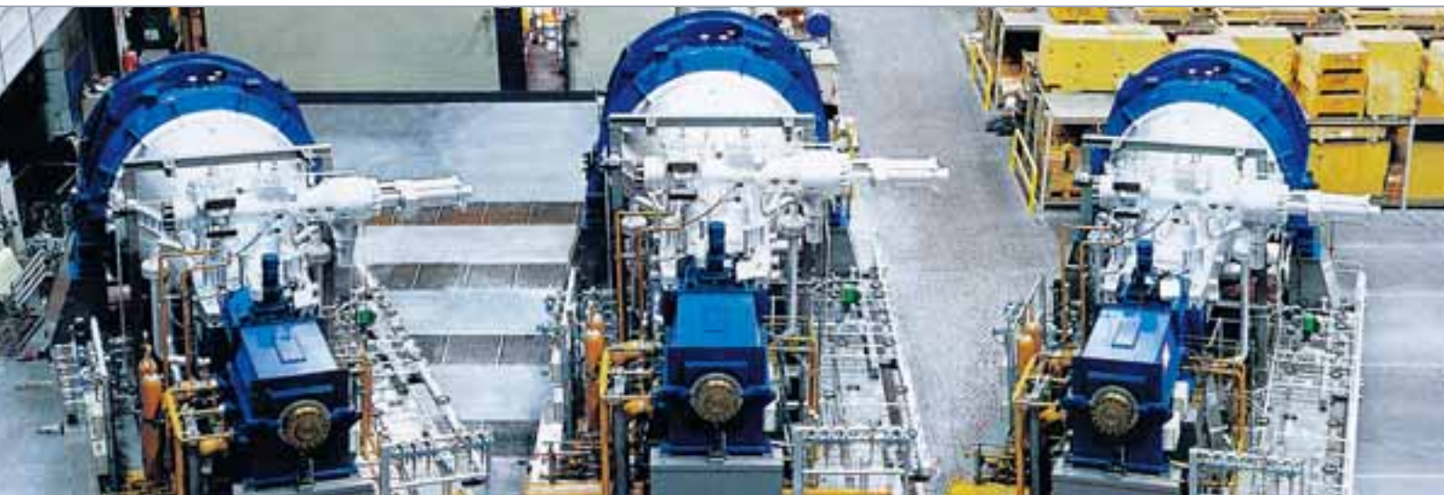
2 Three 38 MW condensing steam turbines for a 300 MWe combined-cycle power plant
