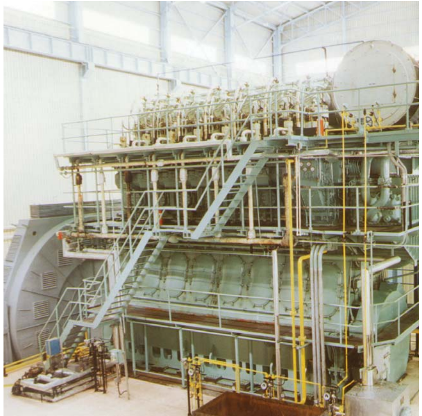
40 MW power plant at Cheju, Korea
